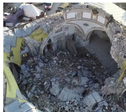
Figure 11. Interior view showing the collapse of the mosque's west wall, while the north and east arches that support the dome remain standing. This figure has been adapted from the “DHA” website [43].
