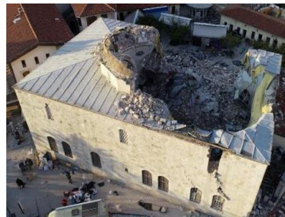
Figure 9. Aerial view of the Habibi Neccar Mosque showing visible shear cracks along the south walls. This figure has been adapted from the “DHA and istockphoto” website [43,44].
