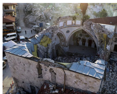
Figure 7. Complete collapse of the minaret and dome of the Habibi Neccar Mosque after the earthquake of Mw 7.7. The debris also affected the adjacent buildings on the southwest side. The figure has been adapted from the “DHA” website [43].
