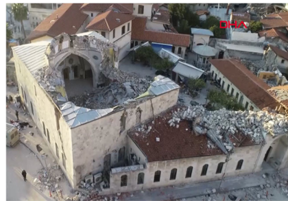
Figure 8. Collapse of the west wall and partial roof failure of the Habibi Neccar Mosque, with debris indicating the fall of the minaret onto adjacent structural elements. The figure has been adapted from the “DHA” website [43].
